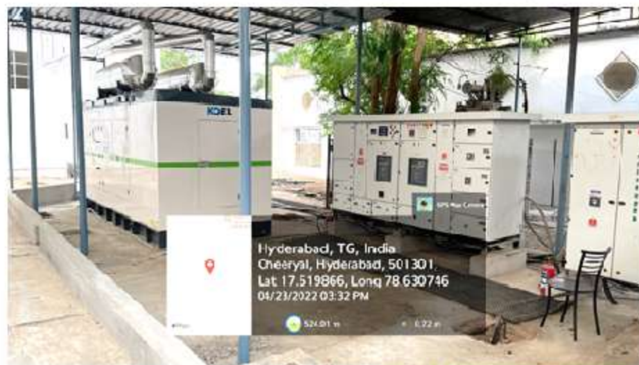
Generator-Power backup facility, GCET
